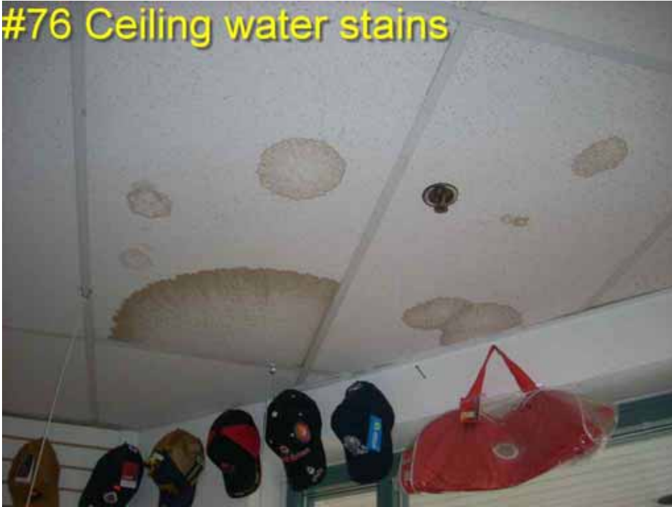
#77 Ceiling water stains
