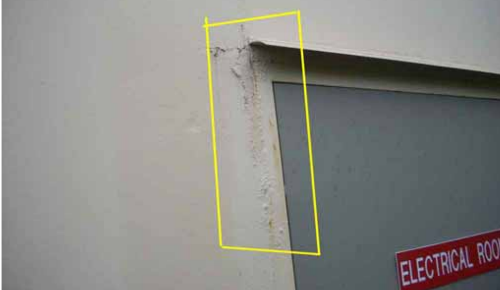
#29 LB box near SE corner has plate open.
