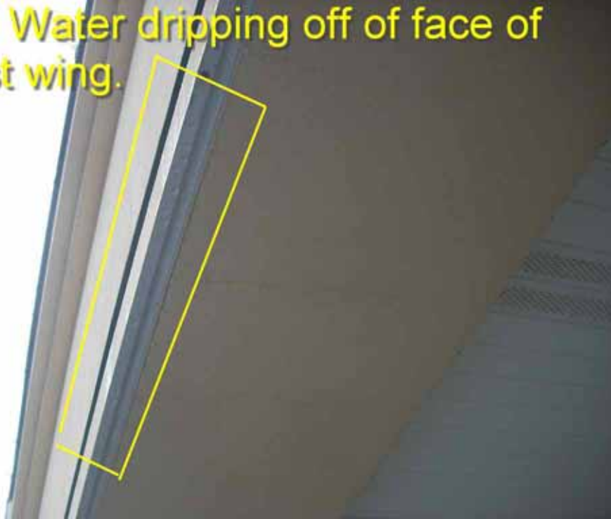
#91 Water stains on soffit area of building 3895
